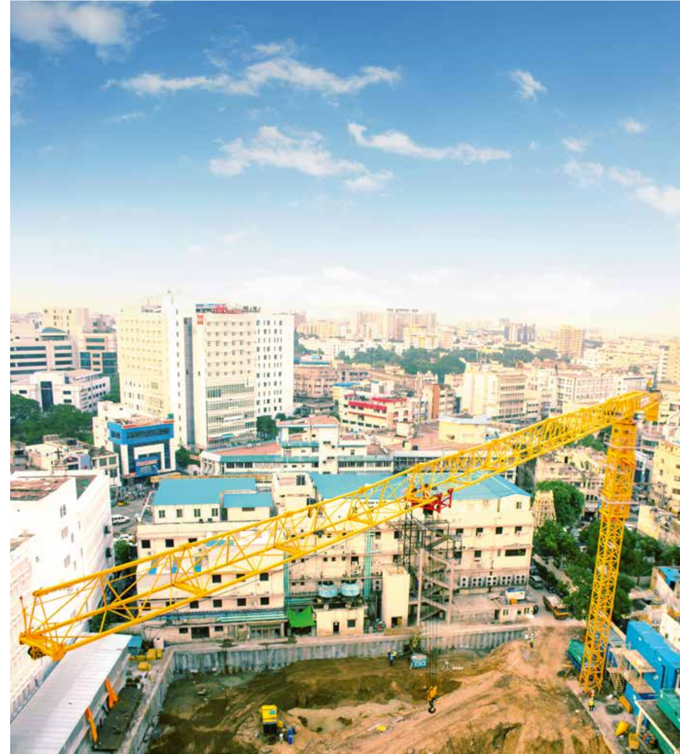
16 ton Tower Crane working at United Insurance Building Project in Chennai for PSK Construction.
