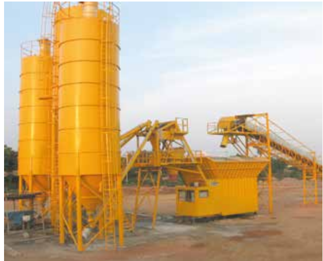
23 year old M1 Batching plant working at L&T Project site
